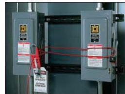
Lockout single or multiple electrical disconnects
