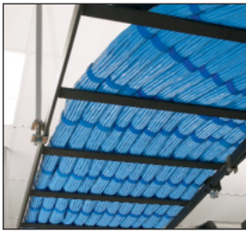
Overhead application Continuous rolls HLS-15R6
