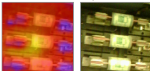
Detect issues with switchgears
