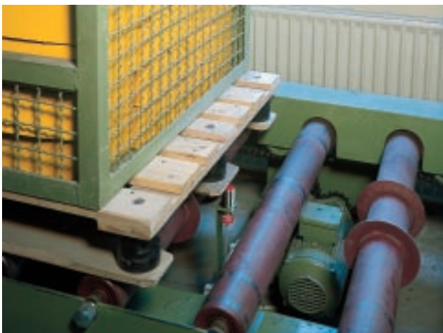
Proximity Sensor in a conveyer application.
